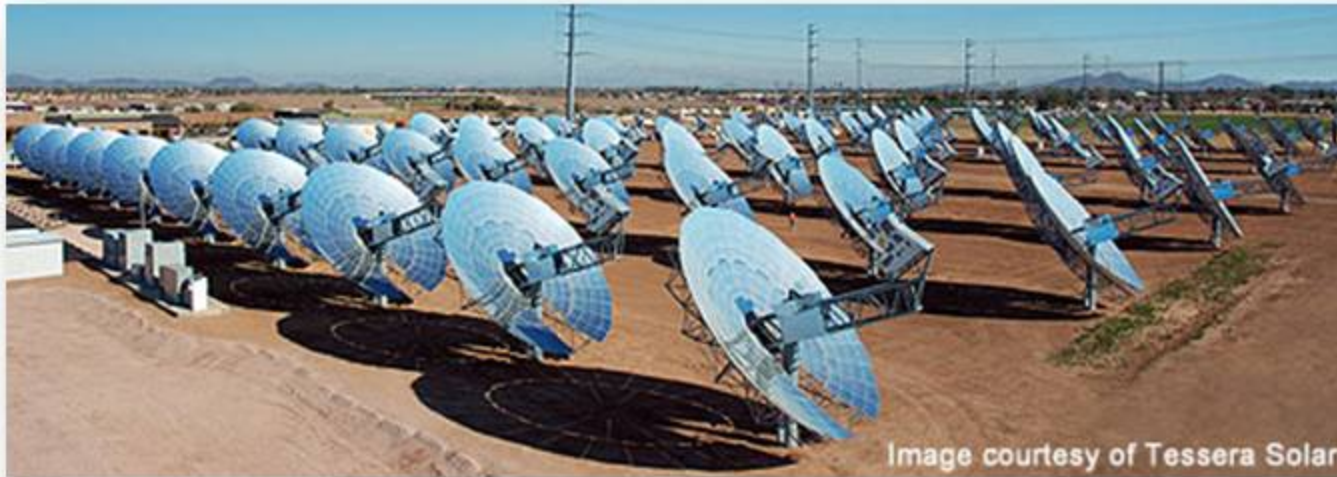
Maricopa solar project by NREL, Arizona, 2011
